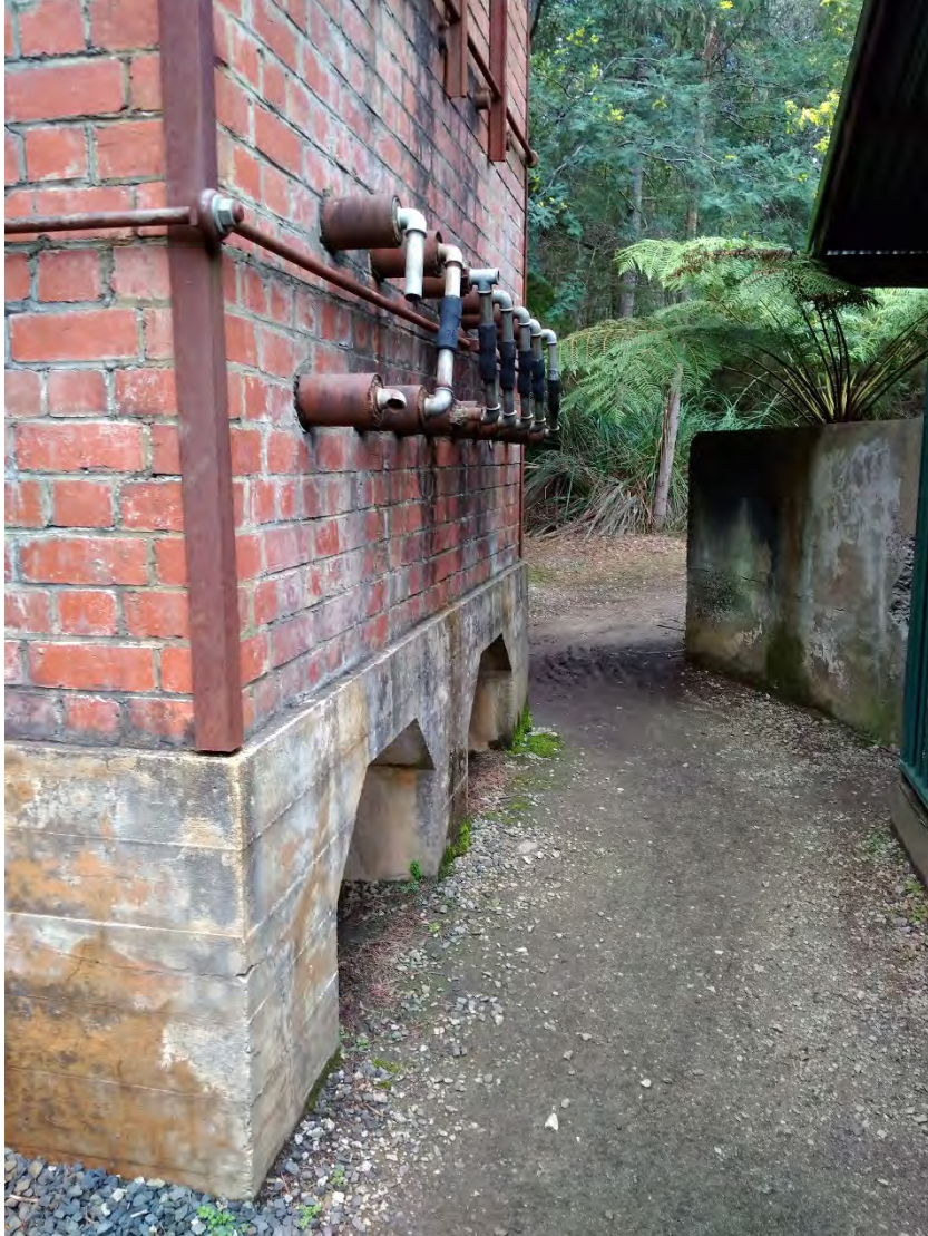
Figure 7. Photo of kiln water pipes on the right (west) side of the kiln, 2018. Photographer, Jane Morton Colbert.
